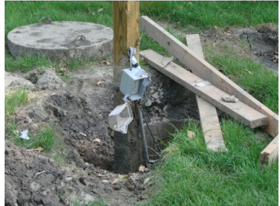
Flood damaged SSTS electrical box
